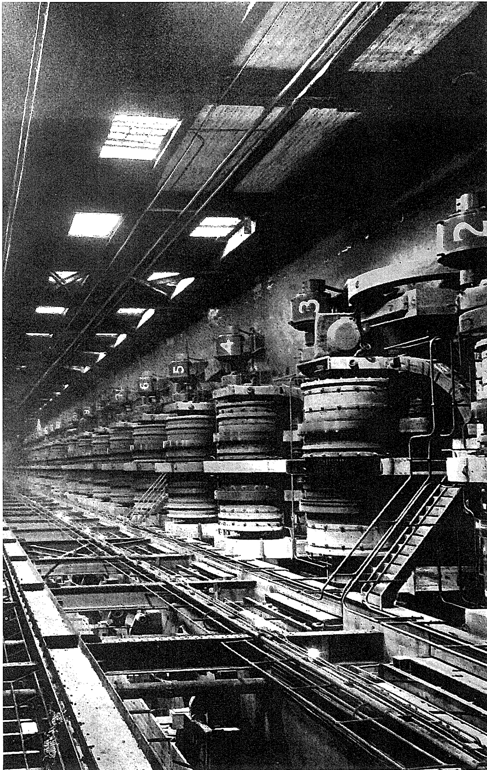
BATTERY OF ROD AND BALL MILLS, COPPER CLIFF CONCENTRATOR
