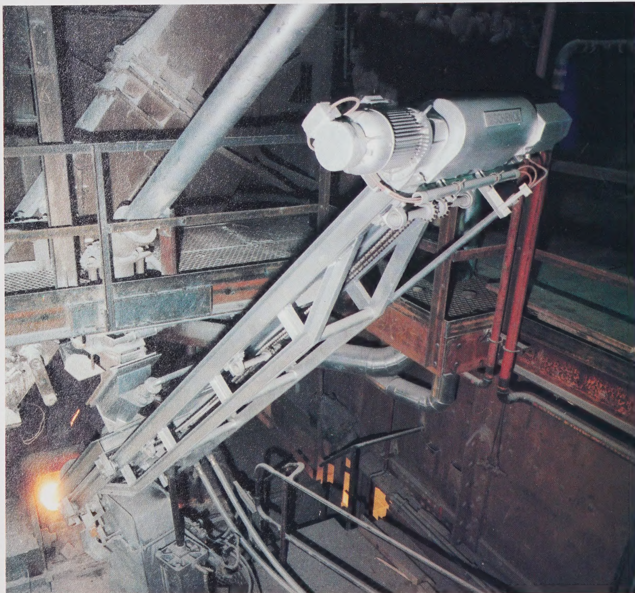
Smelting (top) produces the basic nickel matte from which Inco continues to develop new forms of nickel products for changing markets. One of these products, a granular Nickel Oxide Sinter 75, is now being marketed in bulk for injection by retractable lance (below) directly into furnaces producing stainless steel.
